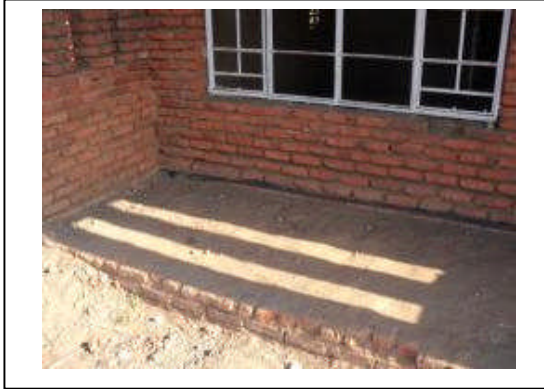
Photo MHC No. 1 – No Floor Slab
