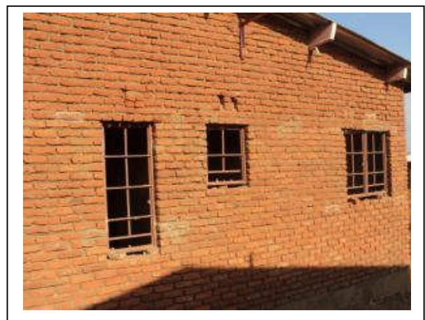
Photo MHC No. 5 – No concrete Lintel over Windows
