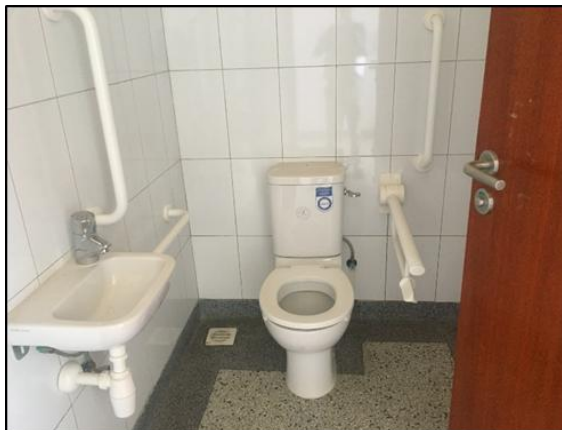
Figure 28: Toilet facilities for PWD's on HEST project
