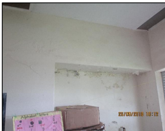
Figure 13: Leakage from poorly renovated roof at NTC Muni
