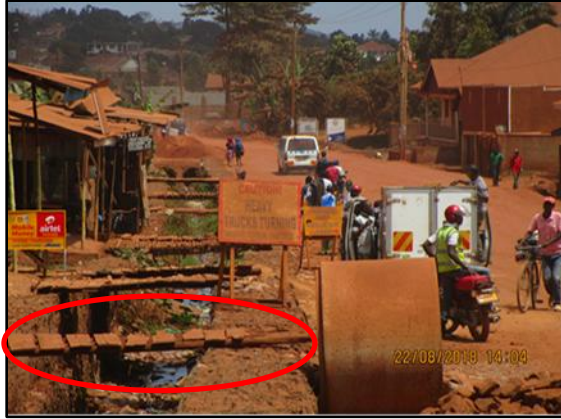
Figure 15: Poorly maintained access at Namasuba road
