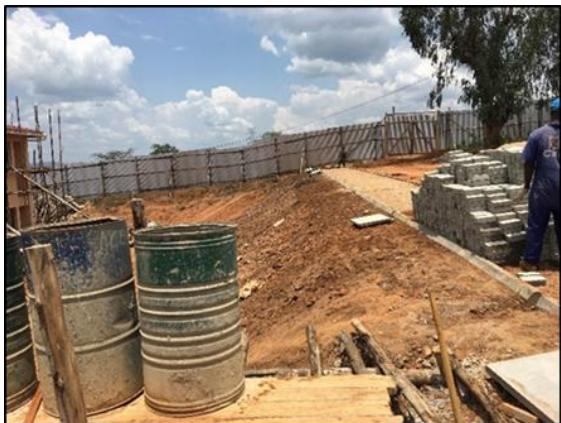
Figure 19: Unprotected embankment (HEST)
