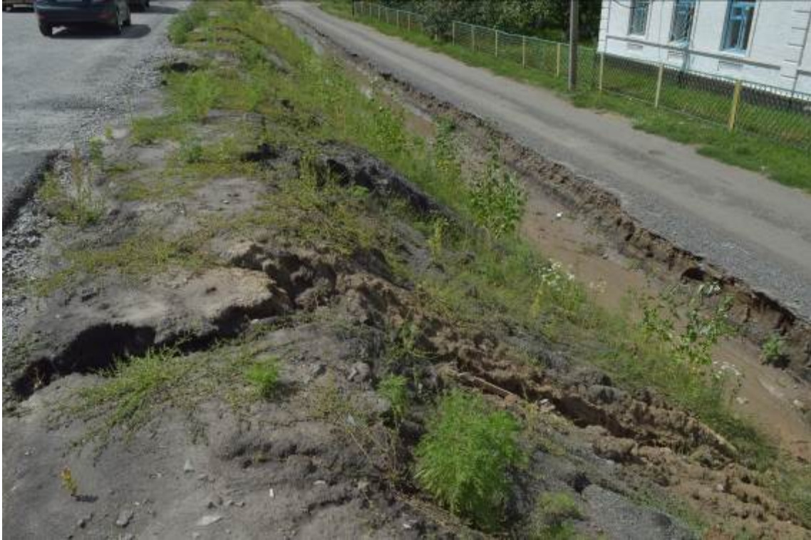
Figure 3 – Washaways in Podil village, km 288+794
