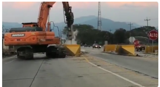
After the PPP was cancelled by the government the tollbooth was removed
